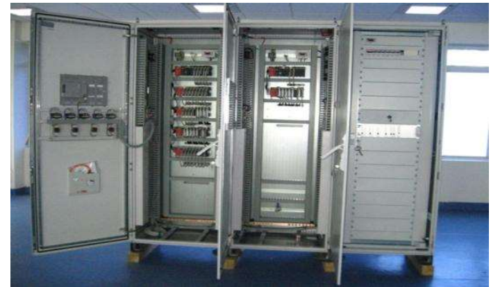
Electrical Control & Instrumentation
